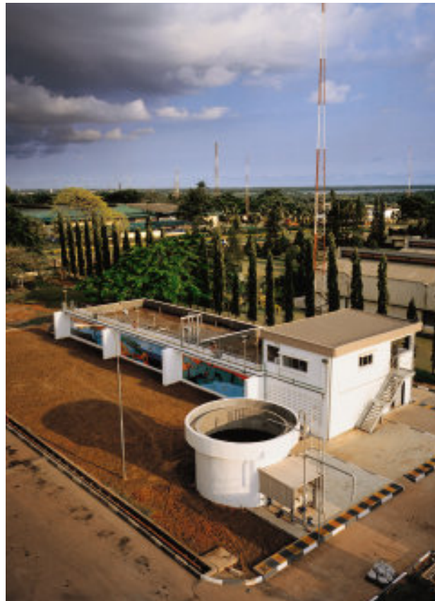
The water processing plant to clean waste water at Nestlé's Agbara factory in Nigeria has won state environmental awards
